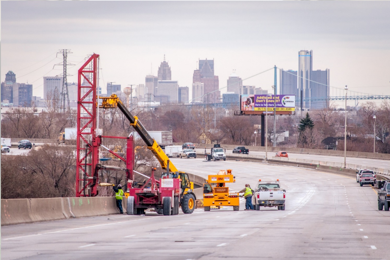
SB I-75 North of Rouge River Installing False Decking Utilizing MOOG Platform
